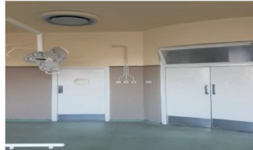
Rehabilitated theatre at Mbuya Nehanda Maternity Hospital that was destroyed by fire
